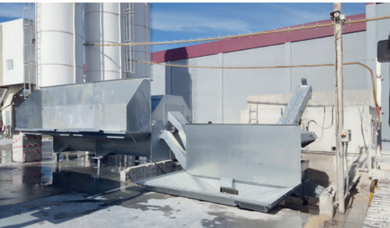
At the Lourel plant, the Bibko ComTec 30 system was installed together with a dosing buffer.
