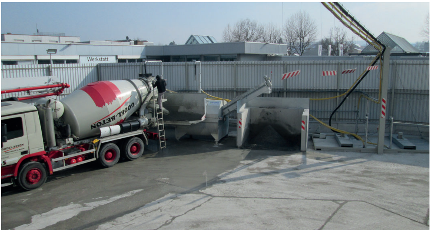
The supplied ComTec 20 system has a recycling capacity of 20 m 3 /h.
