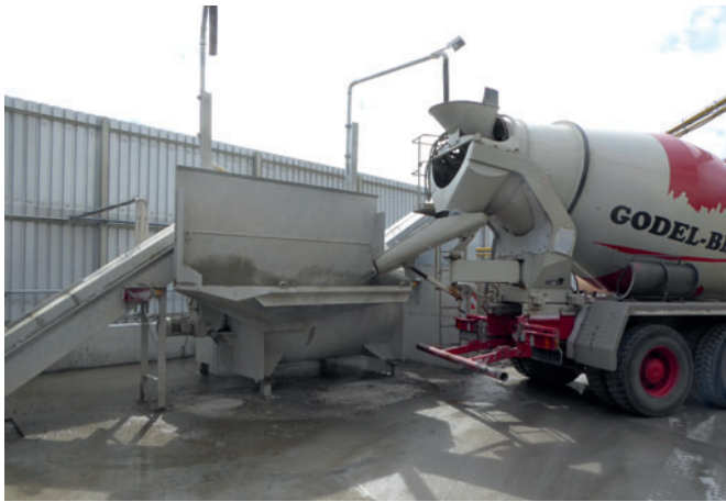
In installing the Bibko recycling system, Godel-Beton is proving acceptance of its ecological responsibility
