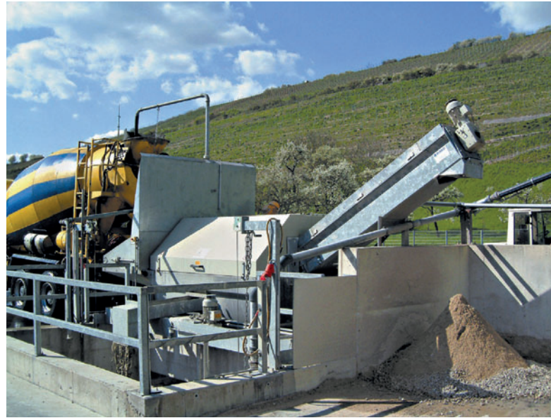
Bibko® residual concrete recycling plant
