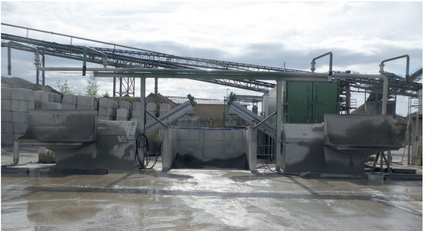
The concept developed comprised two recycling machines including agitators, as well as a chamber filter press.
